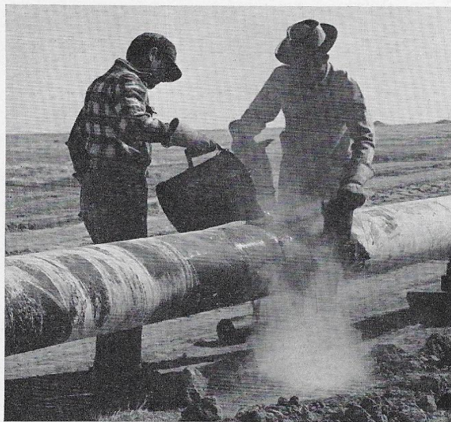
Though most wrapping of the Junction-Oleum line was done in pipe yards, welded joints had to be coated and wrapped at the ditch site. Here hot asphalt and wrap are applied.
