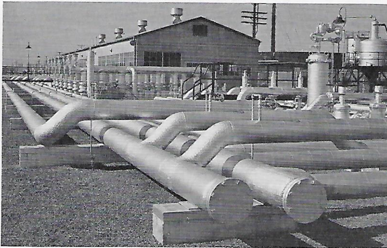
Junction Pump Station, above, is the San Joaquin Valley starting point of Union Oil's new 225-mile pipeline to Oleum Refinery.
