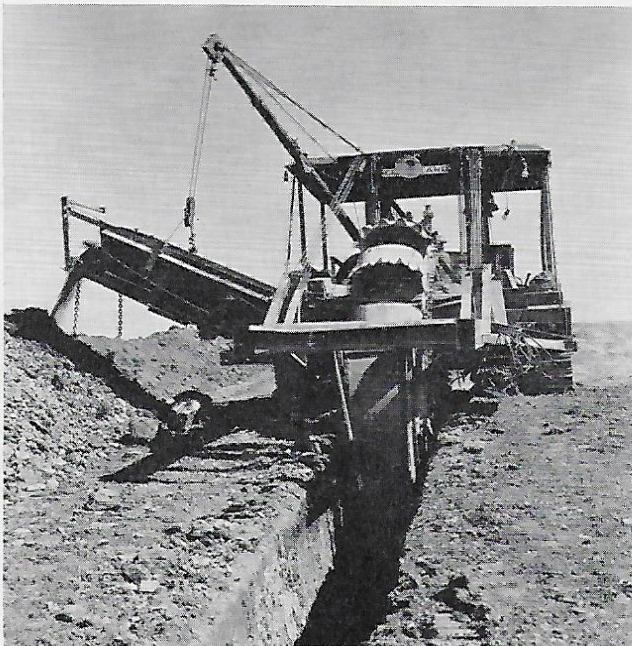
Most of the 225-mile trench was dug by "ditching machines" of this type, which often will bite their way through a mile or more of soil per shift.
