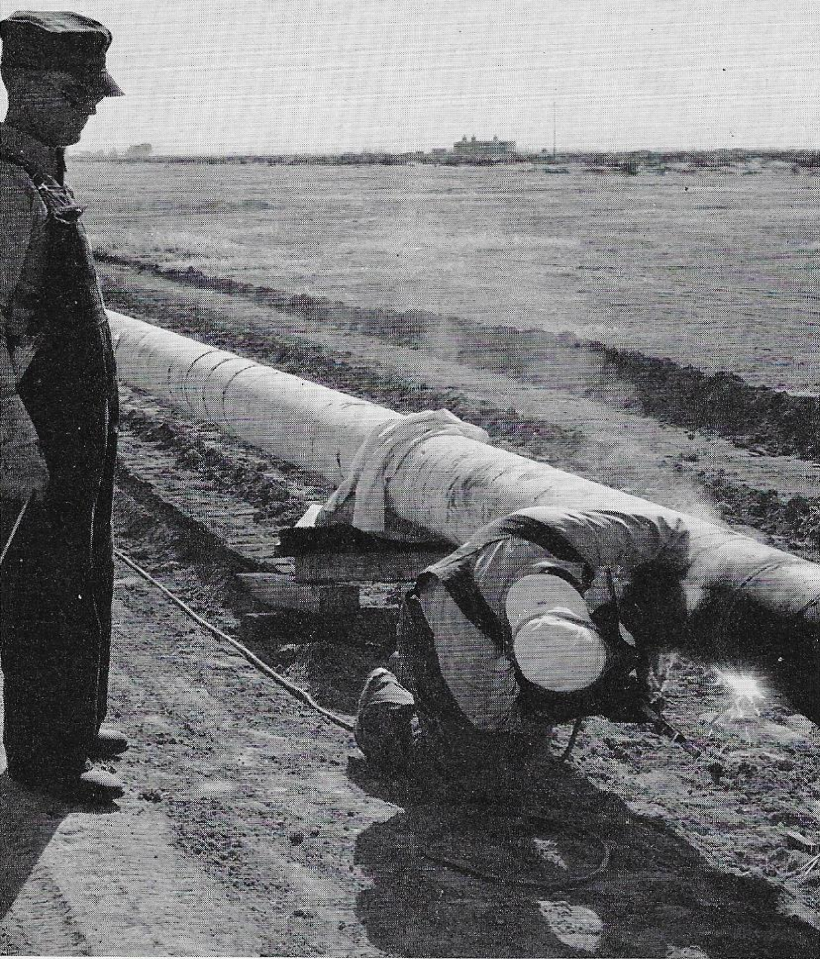
The building of modern pipelines calls for the highest skills of the welding trade. Five or more perfect "beads" seal each joint. Many welders fail to qualify for the job.
